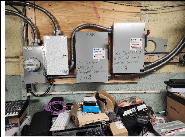
Neighboring units electric panels
