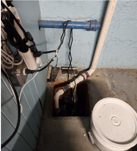
Basement sump pump area
