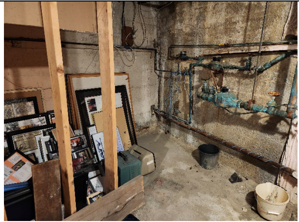
Water meters shared by whole building.
