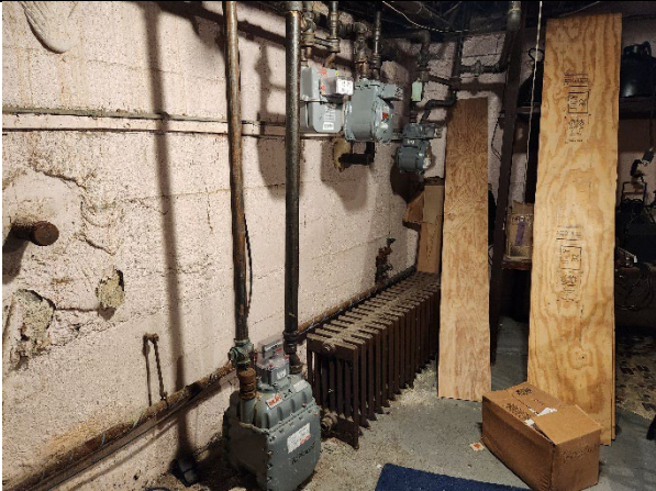
Individual gas meters for building units.
